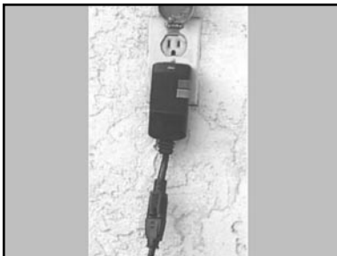
(B) Check to see if the Ground Fault Circuit Interrupter (GFCI) is tripped
